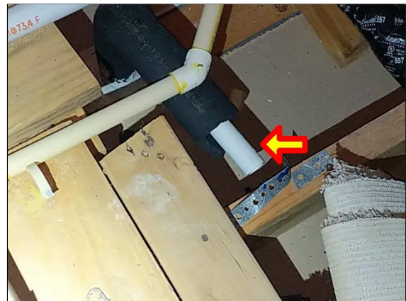
Condensate rain attic not used.
